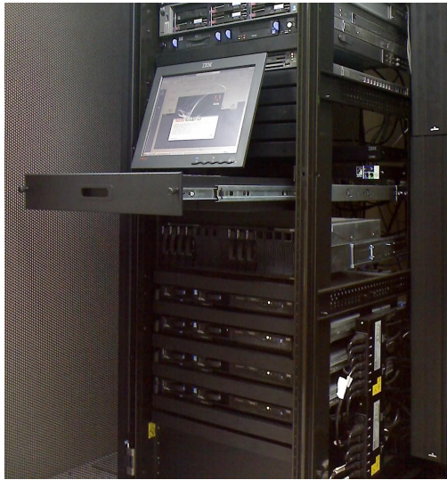
A typical server rack
