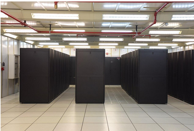
ARSAT Data Center
